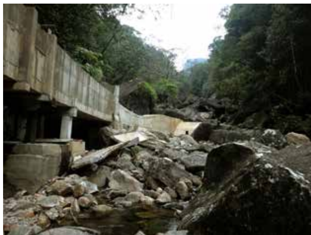
Figure 6. Hydroelectric power plant (note: concrete wall built across the stream and concrete particles dump into the stream).
